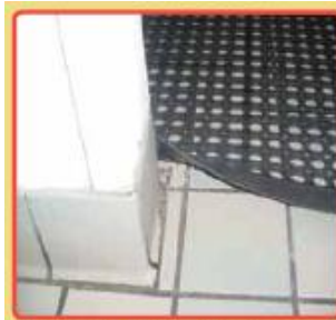
Figure 10.1. Edge of mat is not flat on the ground
