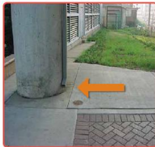
Figure 2.4. Drainpipe routing water onto walkway
