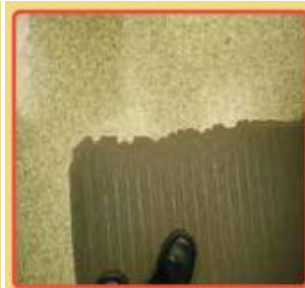
Figure 10.2. Frayed, worn edges on a comfort mat
