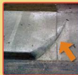
Figure 4.2. Area of sloped pavement that should be highlighted with Safety Yellow paint
