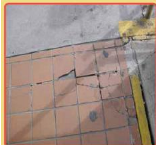
Figure 4.1. Cracked tiles in a walkway outside a hospital building
