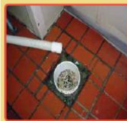
Figure 2.1. Pipe is not aligned properly with the drain causing standing water on the floor
