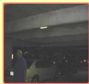
Figure 6.1. Dim lighting in parking area; light fixture is partially obscured by ceiling beams
